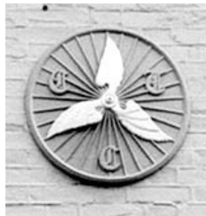
The CTC cast iron sign as it was before someone smothered it in masonry paint.
