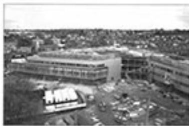
The construction of South New College as seen from the roof of the old College
