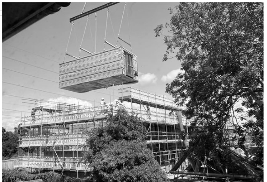
L&G modular units being dismantled at Bristol site earlier this year because of foundations problems.
