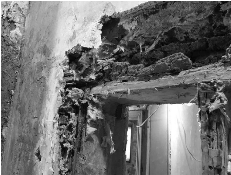
Decay found in the structure.
